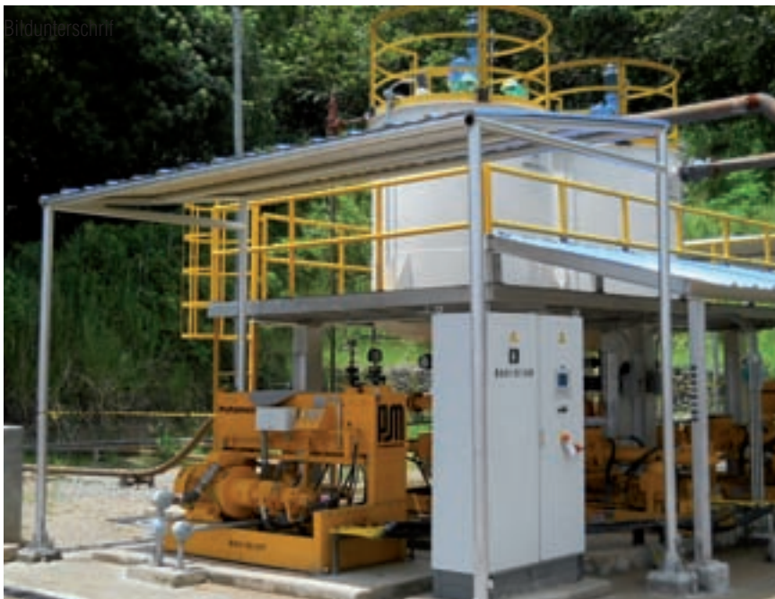
Platform with two pumps
