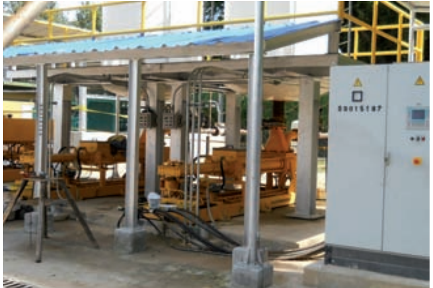
Another platform with HSP 1050 pumps
