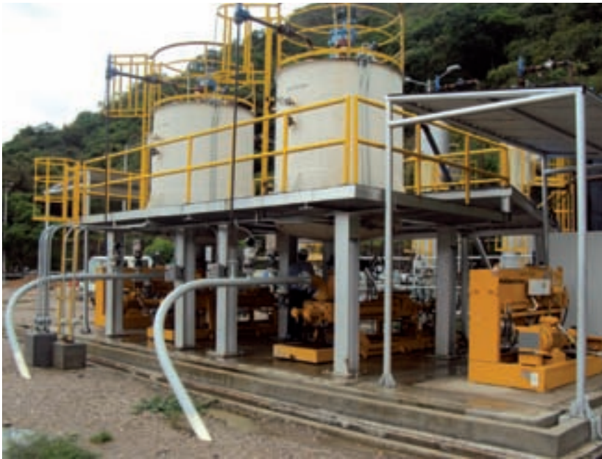
Hydraulic power pack outside explosion area
